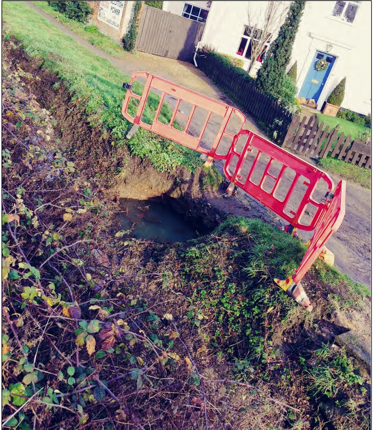
Figure 4-8 - Remnants of attempted remedial works to channel
